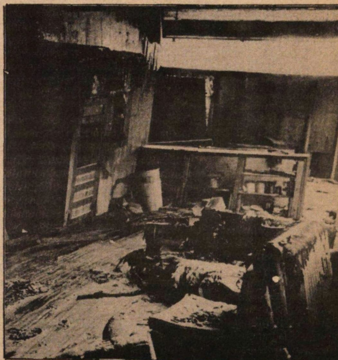
Burned remains of Community Center offices.
